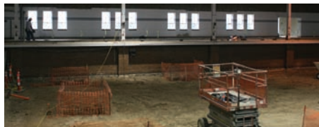
Inside the future weight facility, orange fencing shows footings for the columns that will support the new gym floor that will be built above it.
