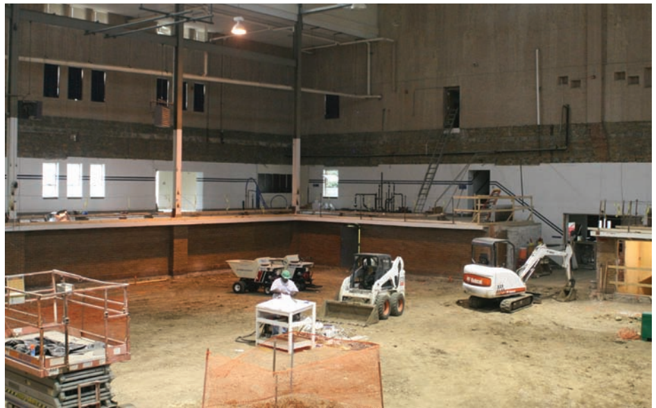
The old north entrance to the field house will become a new glass stair tower and elevator to the upper levels.
